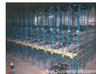
Rack Supported Mezzanine
